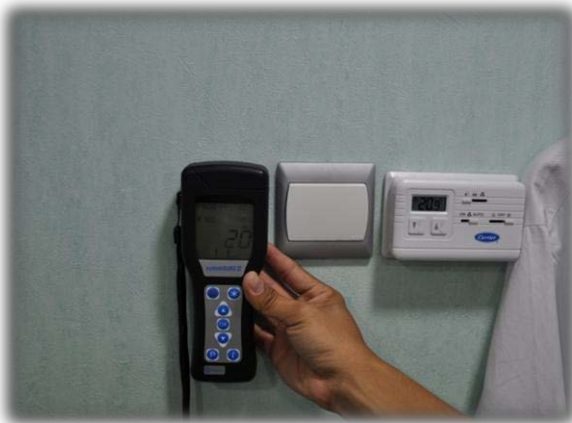
Switches of the Operation room @ 20-caution
